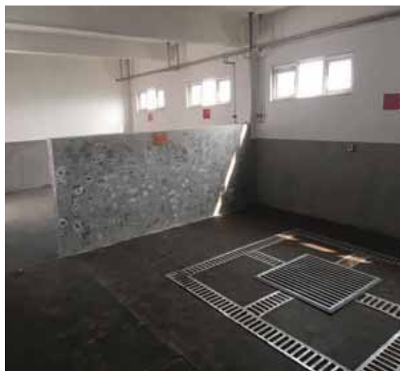
危废暂存间防渗地胶、防渗地漏及托盘
